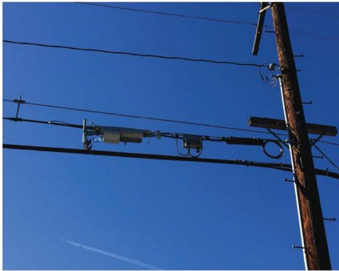
Figure 2. Small Cell and Down-Converter Mounted on a Strand.
