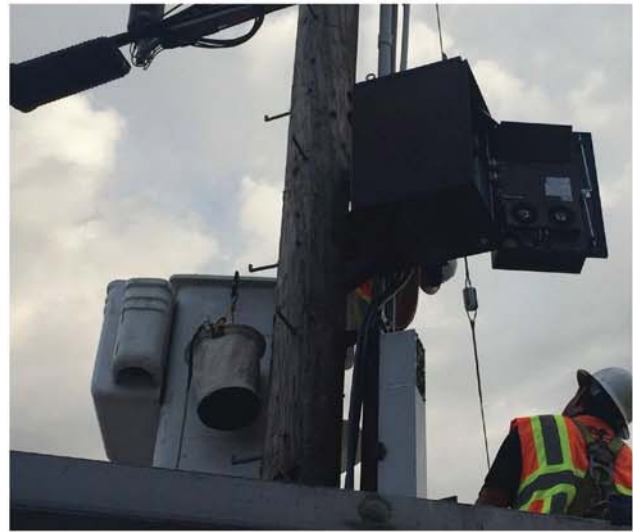
Figure 3A. Remote Power Node Cabinet.
